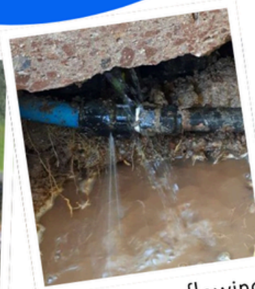
Visible water flowing from underground
